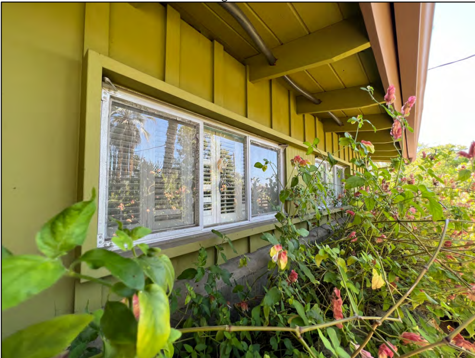
Photo 6: To the far west end of the elevation are three aluminum casement windows. Source: Urbana Preservation & Planning, LLC
