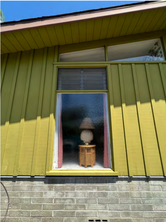
Photo 7c: Based on the Residential blueprints, the elevation was initially supposed to feature two evenly spaced, large rectangular windows, and two louvered windows, to have a more balanced appearance. However, the windows to the right were never installed. Source: Urbana Preservation & Planning, LLC.
