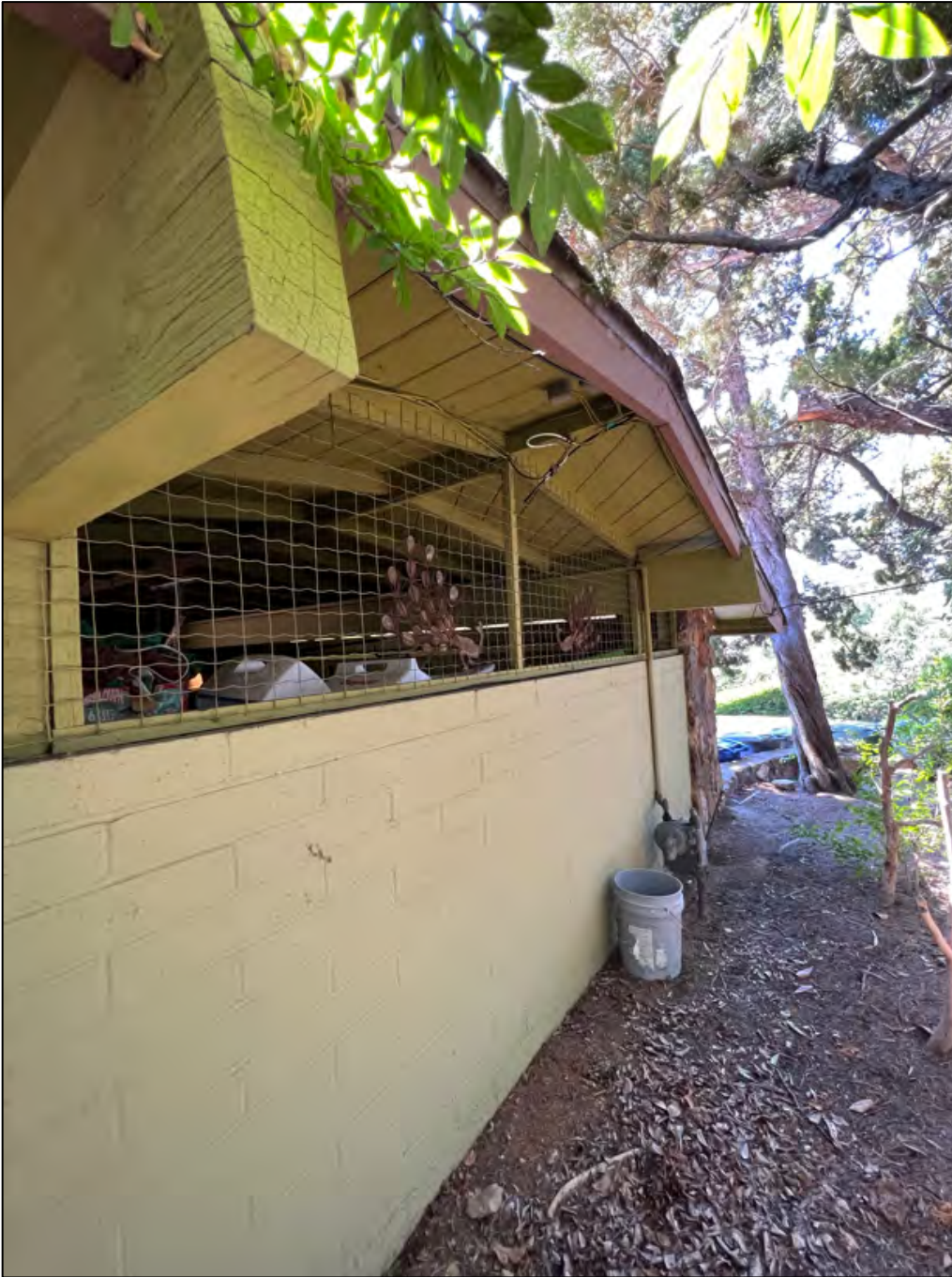
Photo 8b: Detail view of exposed rafter beams and concrete block wall. Source: Urbana Preservation & Planning, LLC.
