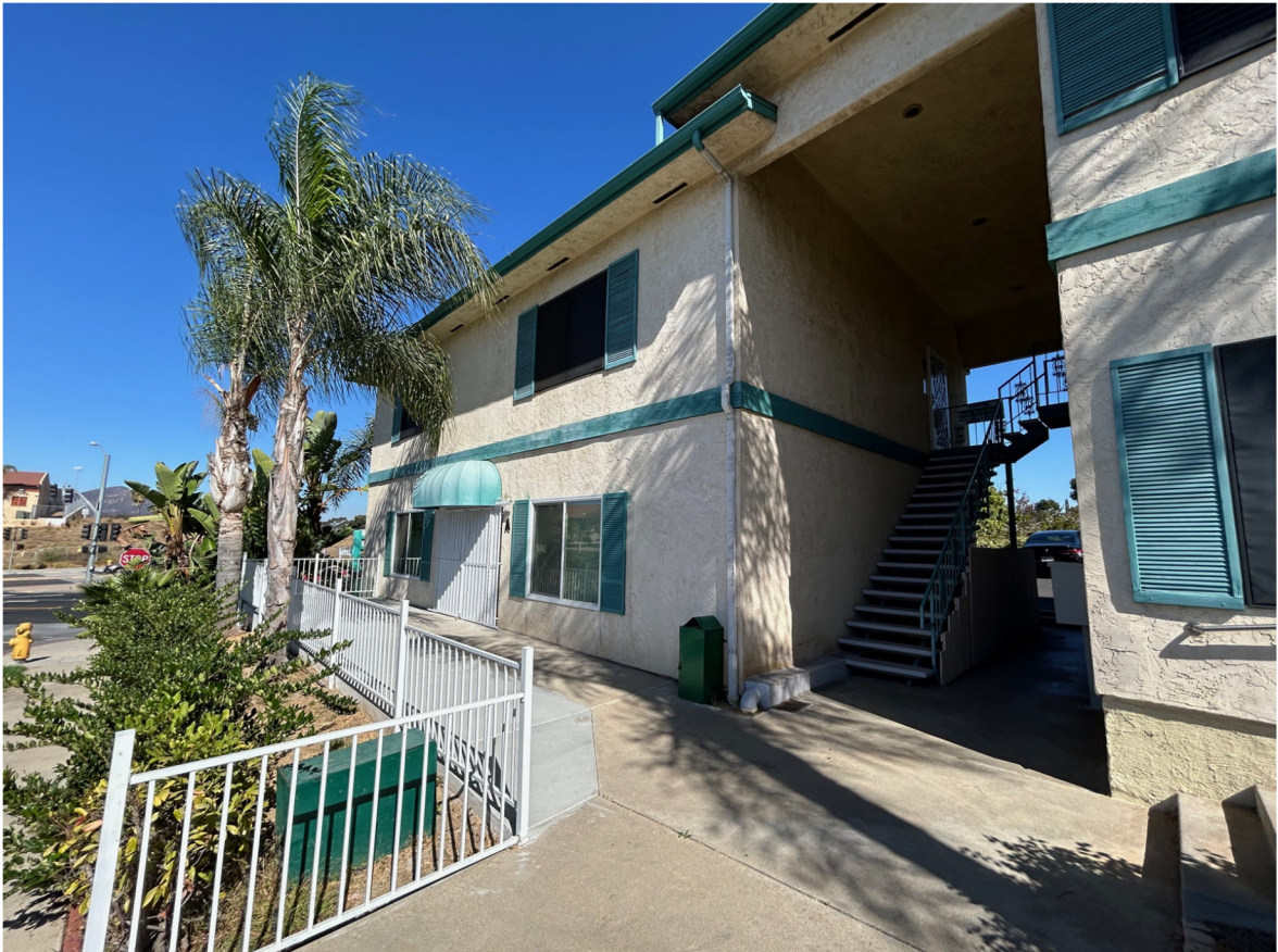
Partial west elevation at the location of the proposed first-floor adult day care center, looking north.
