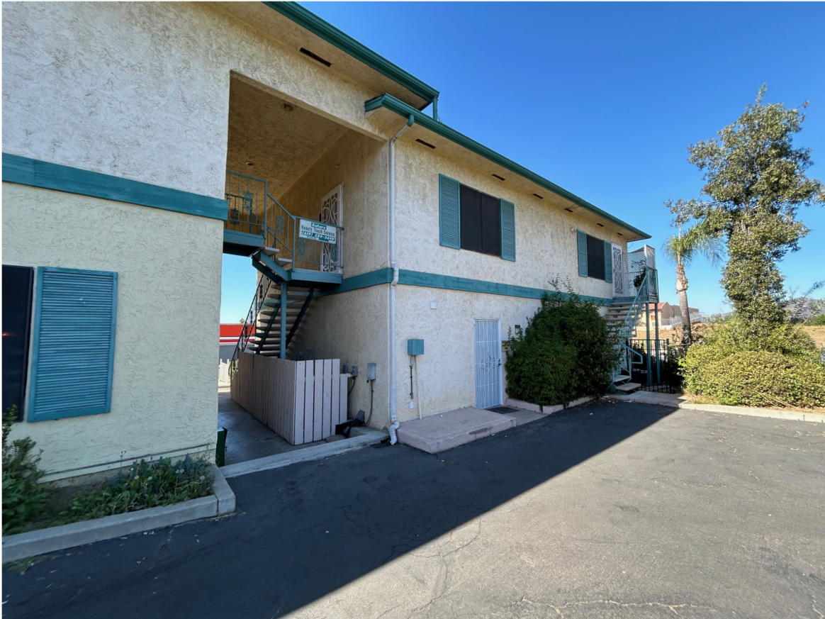
Partial east elevation at the location of the proposed first-floor adult day care center.
